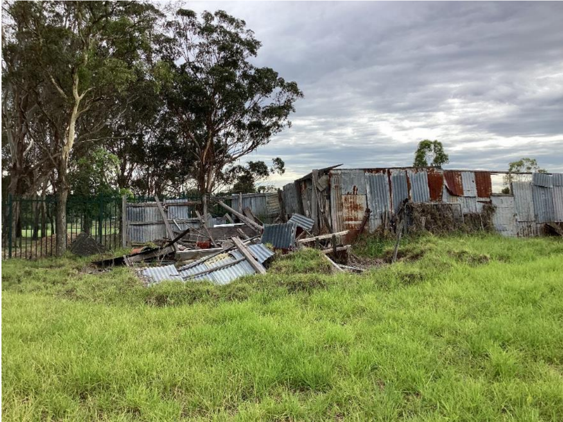
Image 37: Example of dilapidated and partially demolished shed structures on Lot B DP411211 (taken facing north, 25/01/2025)
